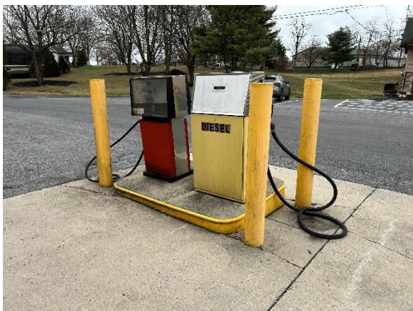
Township Fueling Station
