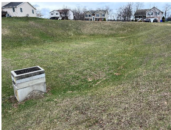
Retention Basin along Hamilton Hills Drive 1
