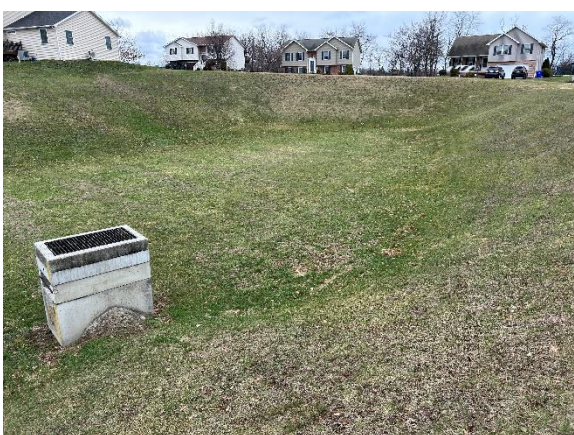
Retention Basin along Hamilton Hills Drive 3
