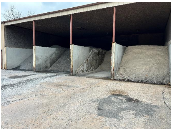
Road Salt Storage
