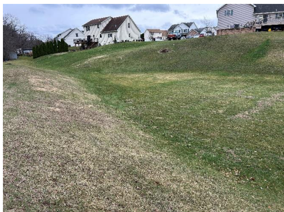
Retention Basin along Hamilton Hills Drive 2
